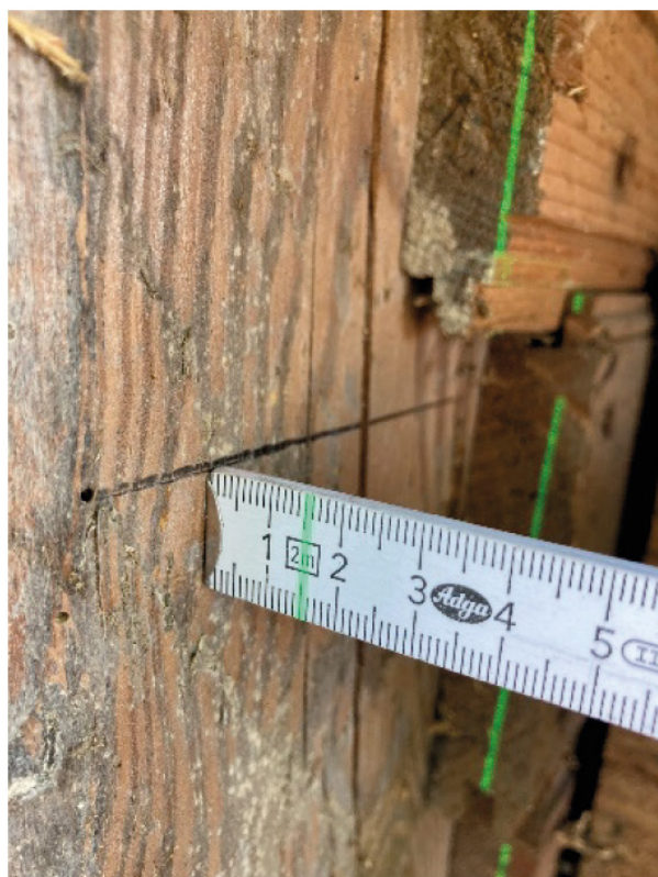
Fig. 5. Photograph taken during measurements of structural element deviations – [photo by A. Kłembokowski]
