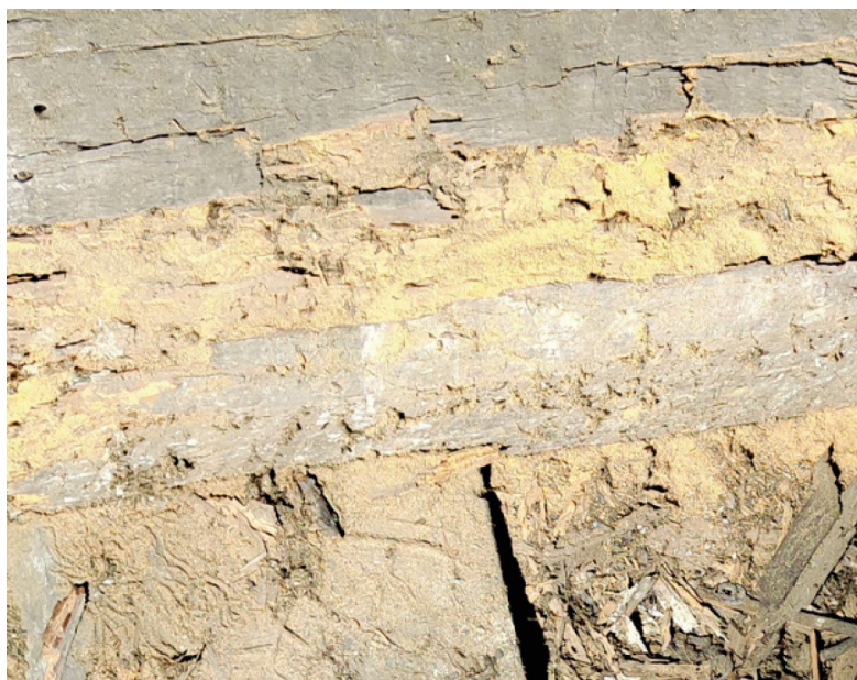
Fig. 3. Example of a biologically deteriorated floor beam – [photo by M. Trochonowicz]
