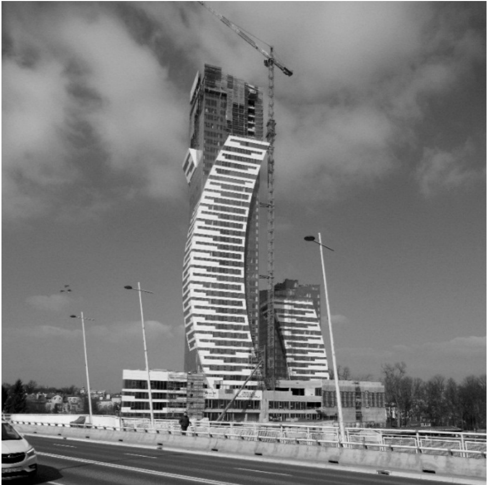
Fig. 16. Olszynki Park in Rzeszów at the final stage of construction. The building will be the tallest in the city and one of the tallest residential buildings in Poland [photo by the author, 2024]
