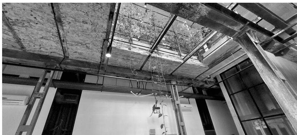
Fig. 6. Main Building of the Żnin Sugar Factory – Using Existing Ceilings as Permanent Formwork for New Construction [phot. author, 12.08.2023]
