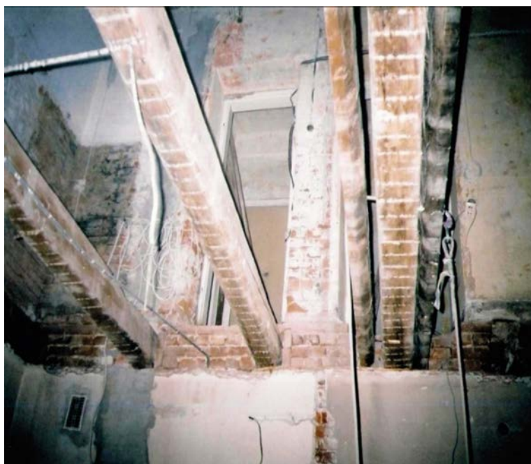
Fig. 18. Residential building located at 17 Stawiszyńska Street in Kalisz, photography from year 2024 [Przemysław Konopski]
