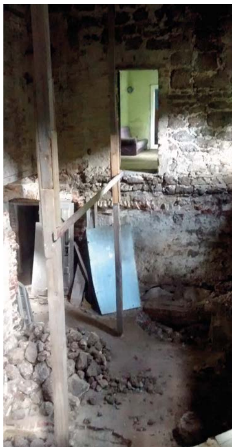
Fig. 12. Manor and farm complex, photography from year 2020 [arch. WKZ Delegation in Kalisz]
