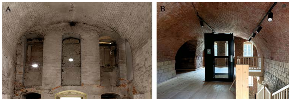
Fig. 31. Interior view of the casemate: 2018 (A); 2024 (B) [Archives of the Department of Conservation of Monuments]
