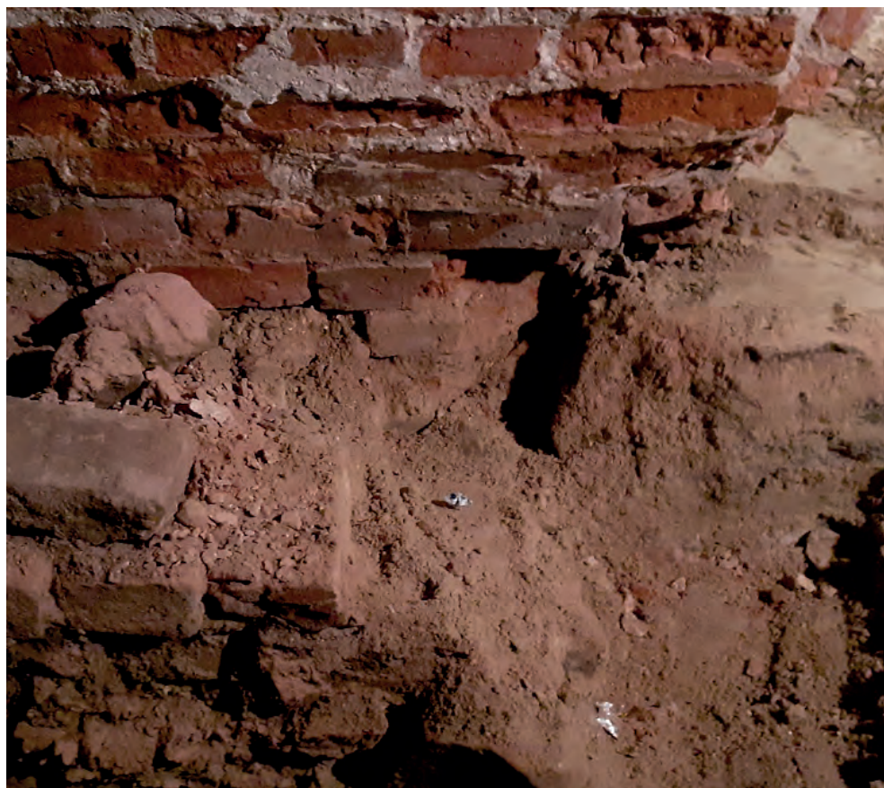
Fig. 16. Condition of foundation walls after removing reinforcing walls and exposing soil layers, photo by A. Kieliszek
