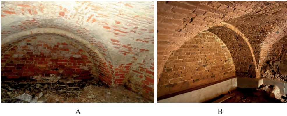
Fig. 23. Brickwork before (A) and after (B) conservation work, 2022, photo by B. Szostak
