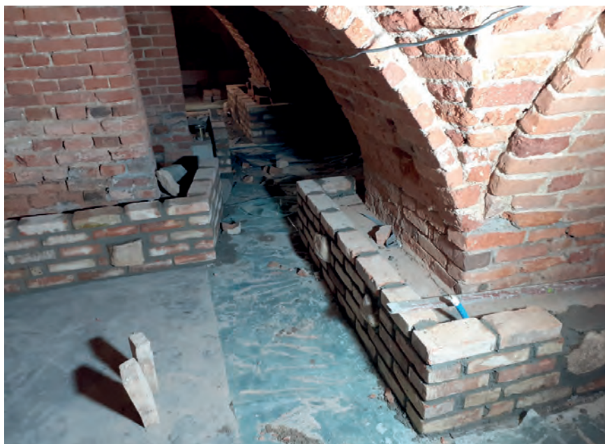
Fig. 22. Crypts during finishing work – covering the reinforced concrete perimeter beams with reclaimed bricks, photo by A. Kieliszek
