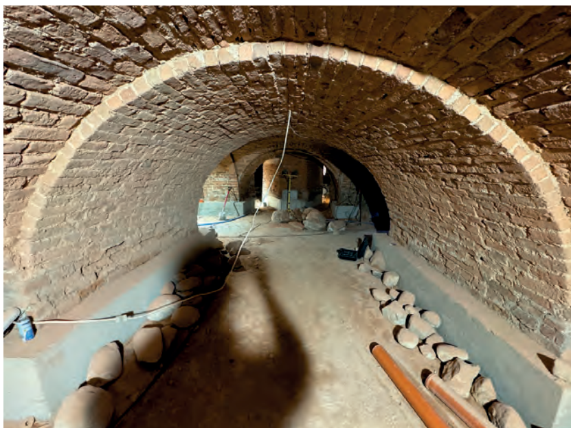
Fig. 19. Crypts after installing the perimeter ring beam and underpinning the foundations, photo by B. Szostak
