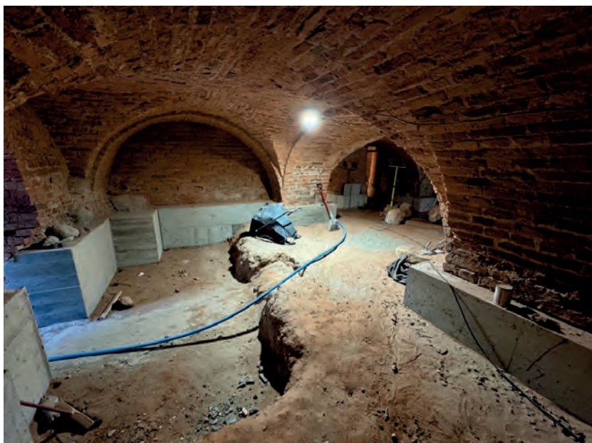
Fig. 18. Crypts after installing the perimeter ring beam and underpinning the foundations – northern corner, photo by B. Szostak
