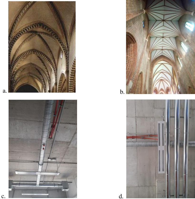
Fig. 2. Structural elements of the vault ribs as a detail in Gothic churches (A, B) [photo: author]; elements of the installation of the building as a detail in a contemporary building (C, D) [photo: A. Leśniak]
