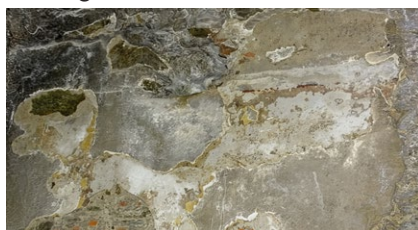
Fig. 25. Plaster, casemate no. 12
