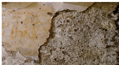
Fig. 24. Plaster, casemate no. 3
